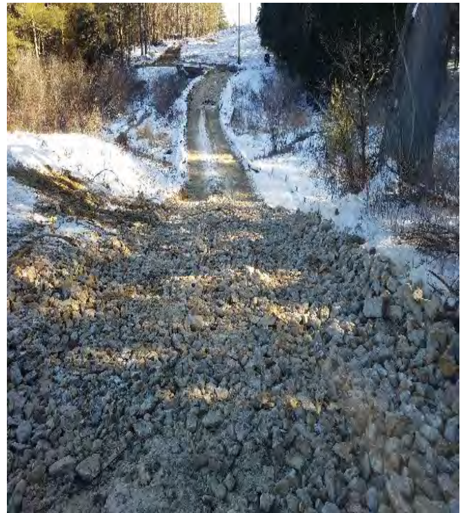
Fig 4: Stone added to access road slope between Strs. 51 and 52. Either side of DS 46. Viewing east. (12-19-19).
