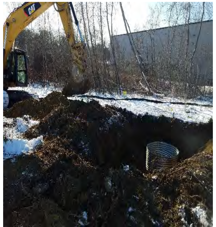
Fig 8: Excavating and setting foundation cans for Str. 141. Soil is used as backfill around can. Viewing south. (12-20-19.)
