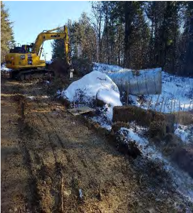
Fig 7: Hammering ledge at Str. 55. Viewing east. (12-19-19).
