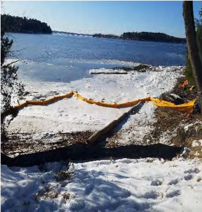
Fig 9: Silt curtain installed at Gundalow landing / east side of the Bay. Viewing west. (12-20-19).
