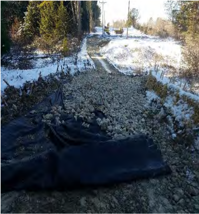
Fig 5: Adding stone to access road slope between Strs. 51 and 52. Either side of DS 46. Note geotextile fabric. Viewing west. (12-19-19).
