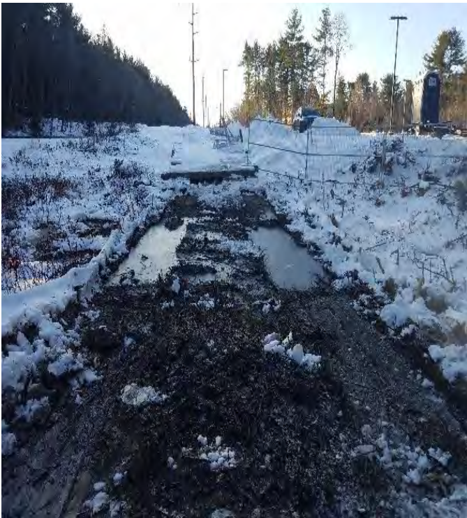
Fig 3: Timber mats removed from wetland DW79. Will restore in the spring. Viewing south. (12-19-19).
